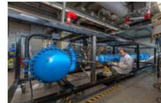
Thermo-acoustic heat pump pilot
